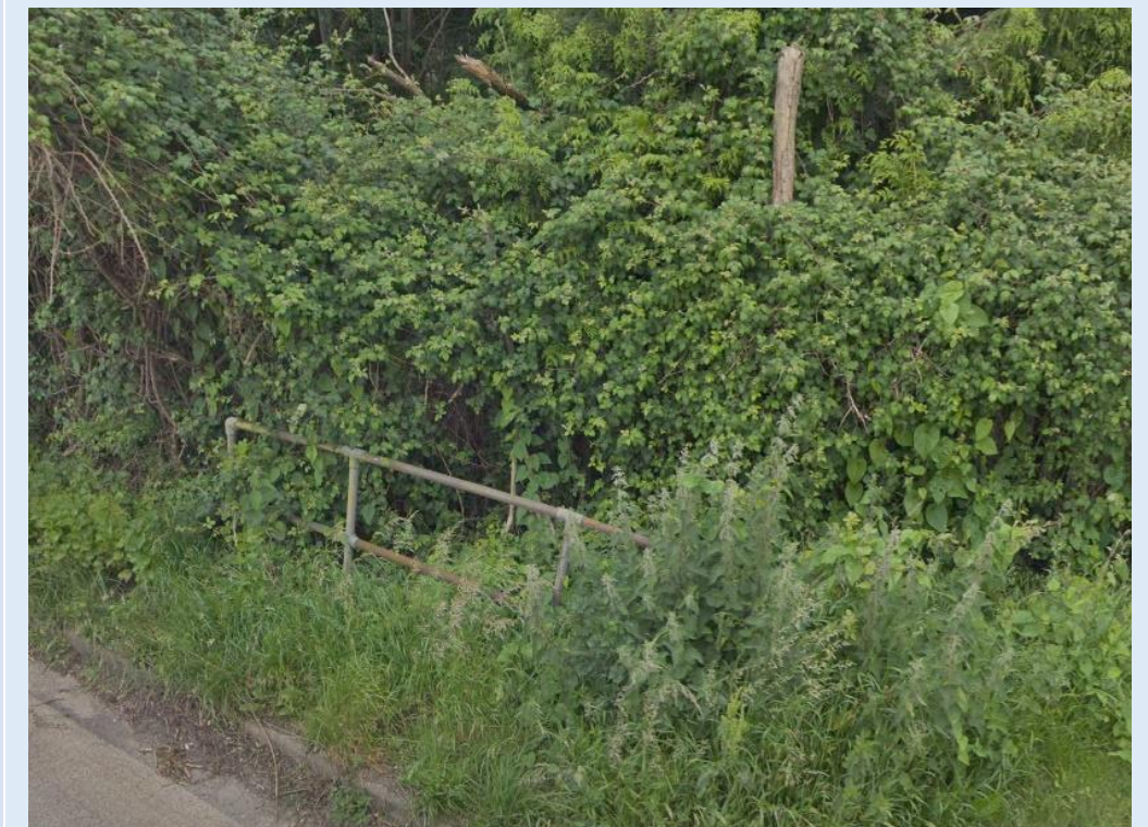
3) View of headwall outfall of culvert on south west boundary of Onshore Order Limit
